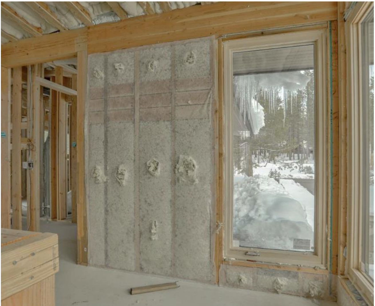
Figure 33: Havelock Wool healthy indoor air residential insulation. 106
